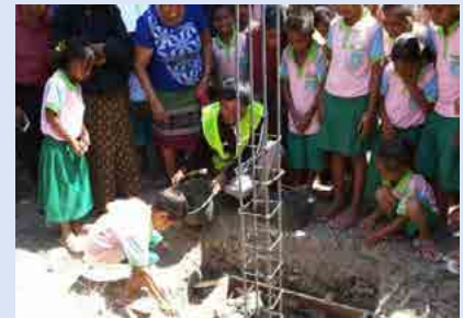
East Timor: First stage of the school reconstruction in the remote district of Abafala
