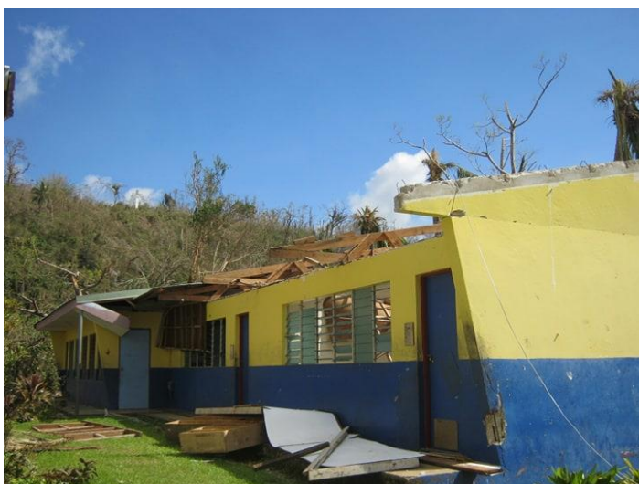
Tropical Cyclone Harold damage to St Michel Technical College
