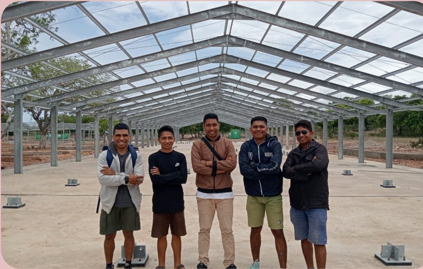
Br Filomeno, Br Dionisio, Br Julio, Br Jacinto and Br Adelino at the Marist School Lautem construction site.
